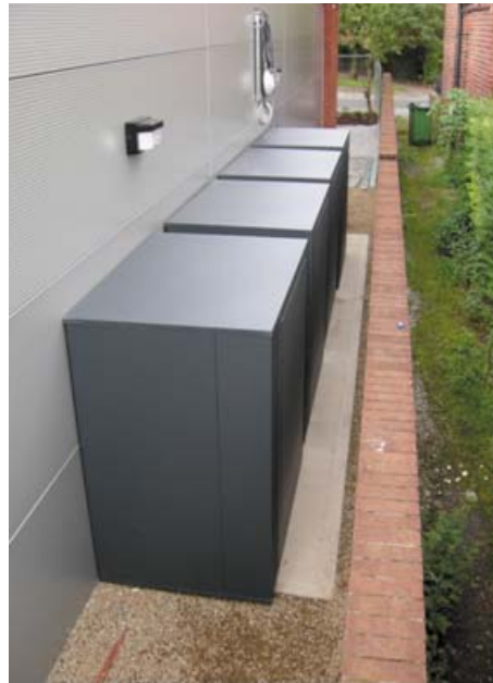
AC units were enclosed in situ using ENVIRON MODULA acoustic ventilation enclosures. An overall noise reduction of 25dB(A) was achieved at source. Install time 5 hours.
