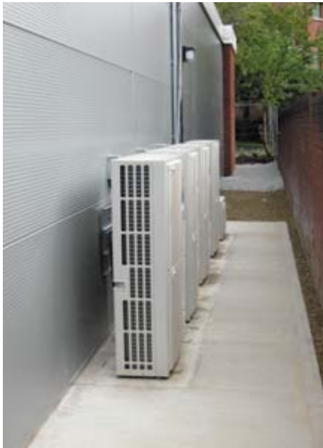
4 NO MITSUBISHI TWIN FAN MR SLIMS at rear of store.
